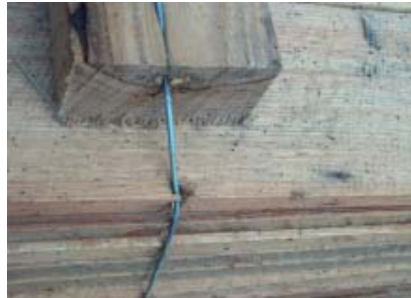
Figure 5.14. Undesirable: No corner protectors
